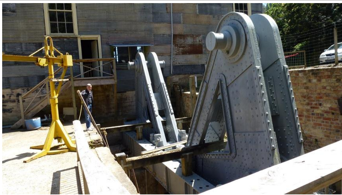
Trevor Burnnand dwarfed by the pump workings at the Pumphouse in Thames
