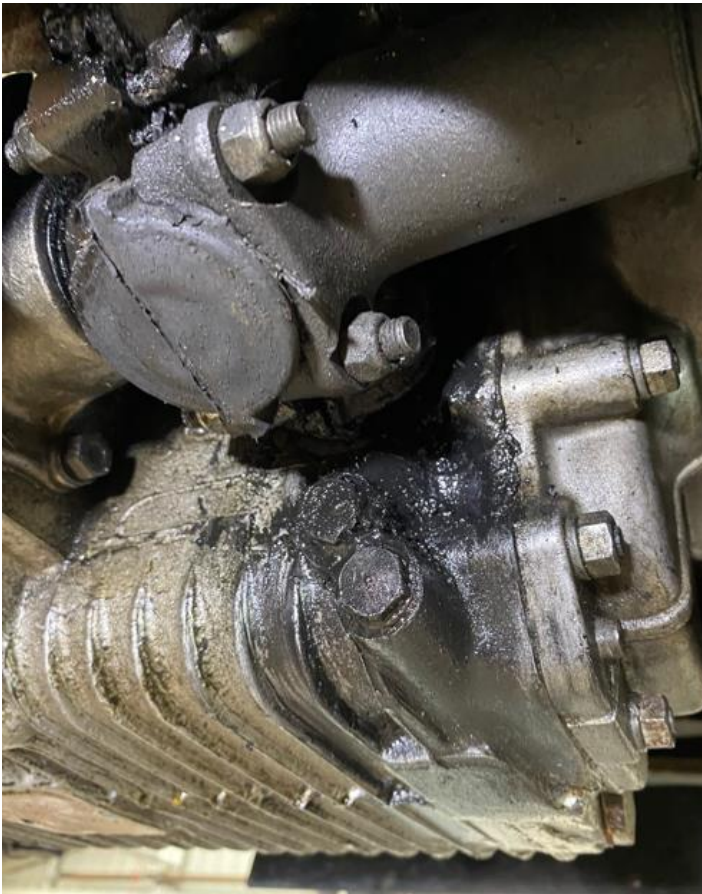
Sign of trouble coming – oil and rubber sprayed onto the gearbox housing
